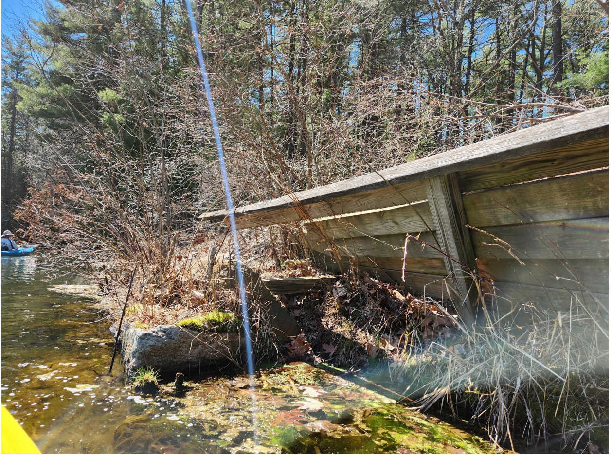
Area 3 - east side is across from boat ramp and has damage - vandalism.
